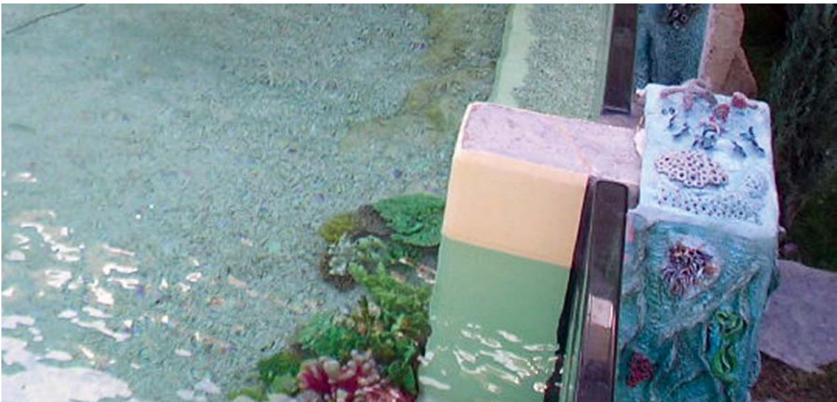
The T-shaped mullions here, which are oversized for aesthetic reasons, allow for sufficient expansion, contraction and minimal deflection of the R-Cast® acrylic panels that allow visitors to look directly into the swim reef at this resort.
